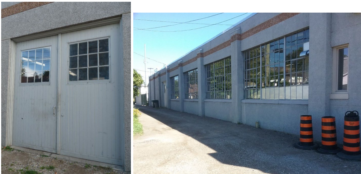
Exterior of the wood doors on the north facade, photographed in September 2016
