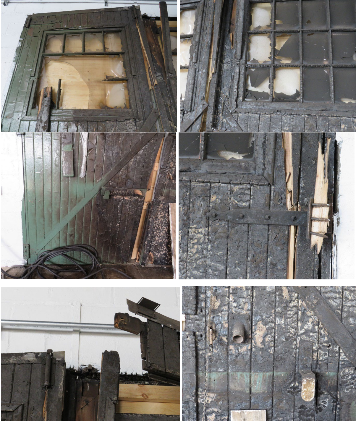
Close-up details of the fire damage to the interior of the wood doors, photographed by Administration in February 2022
